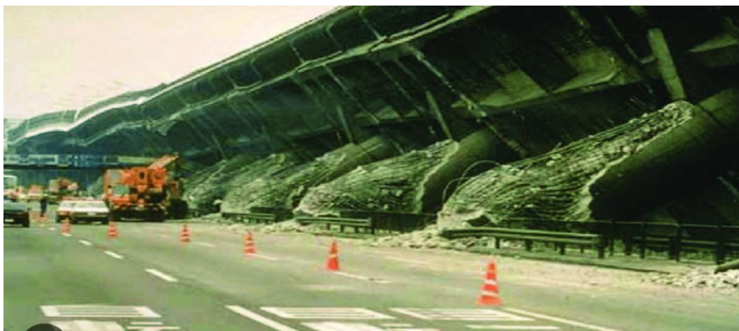
Figure 3. 1995 Hyogo-Ken Nanbu earthquake. Higashi-Nada viaduki
