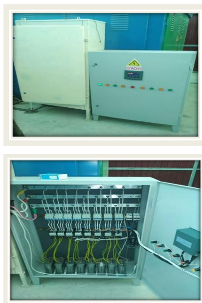
Figure 3: General view of the installation of reactive power compensation capacitors in a feed grinding shop
